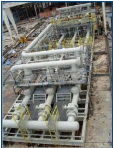
Gas USM Metering Skid
