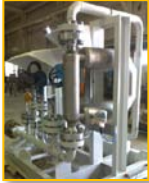
Wet Gas Wellhead
