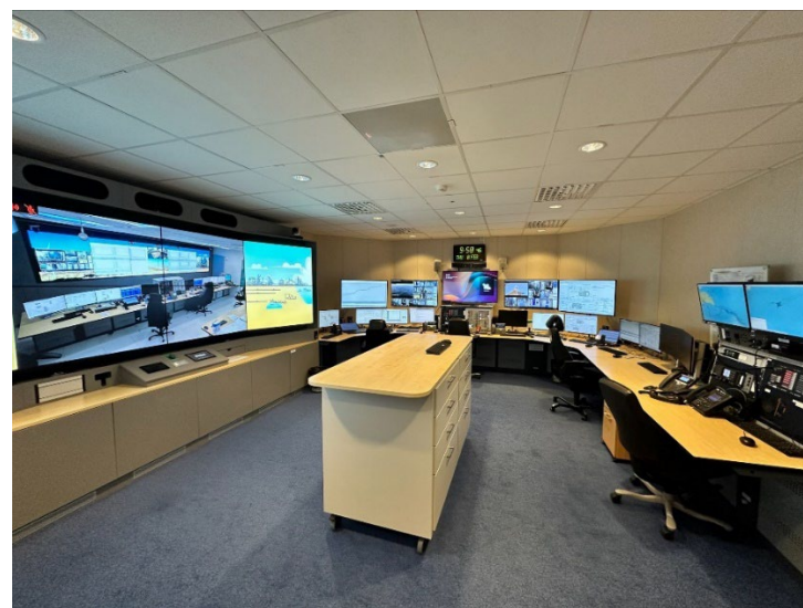
Control Room - unattended
