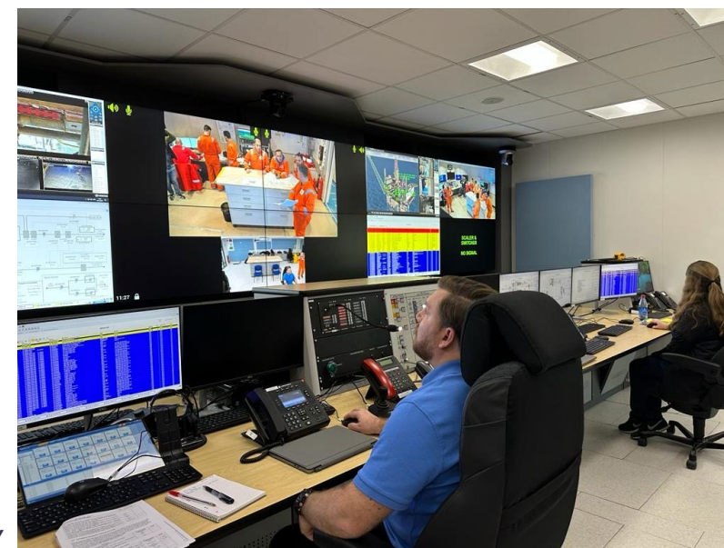
Permanently attended Control Room
