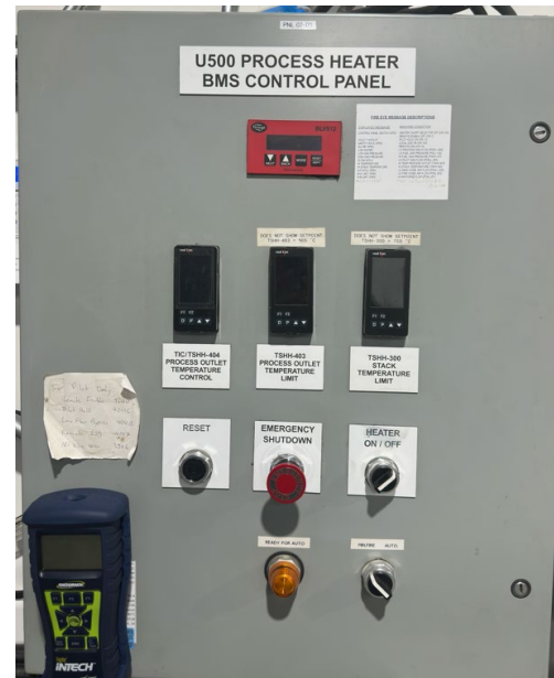
Heater Control Panel
