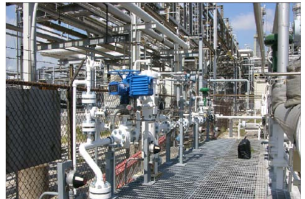
Metering skid with Micro Motion ELITE meter installed for critical phase ethylene custody transfer
