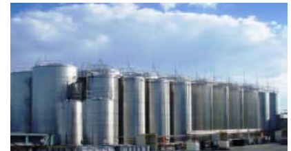
Taller tanks but in smaller diameter Due to limited land available
